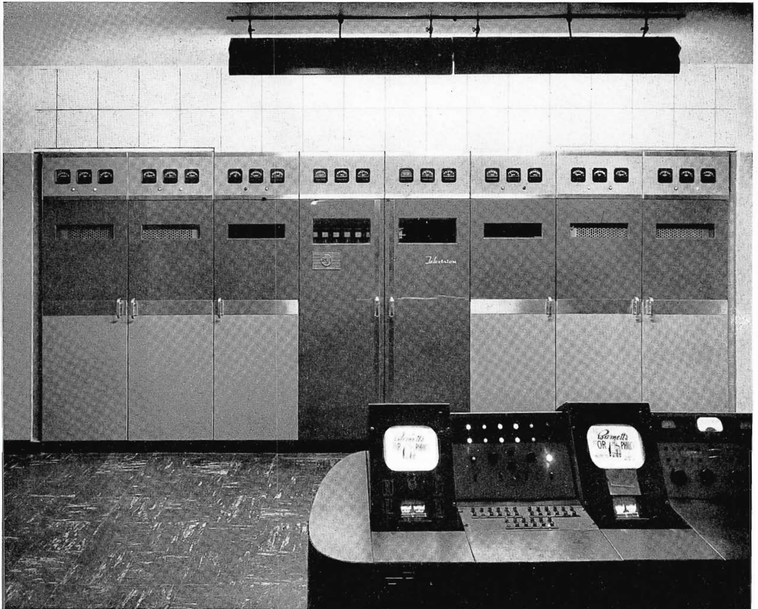
FIG. 18 (above). Front view of the neat, flush-mounted arrangement of the WDSU-TV, RCA TT-5A Transmitter.
